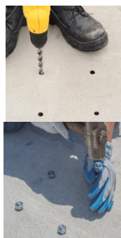
STEP 2: Drill for holes as shown 1/2" wide hole 4" deep and hit down the anchor bolts (1/2" x 4") with a hammer. Then take off the nut before you place the metal anchor ( note: for wood deck use lag bolt ).
