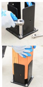
STEP 3: Place and attach metal anchor to concrete with anchor bolt (1/2" x 4") and place the post.
